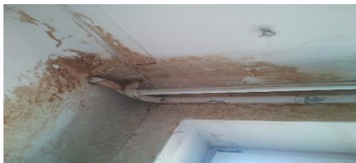
Figure 4 – The microbiological corrosion in industrial building
