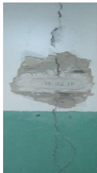
Fig. 2 – Chalky screed state after pile installation
