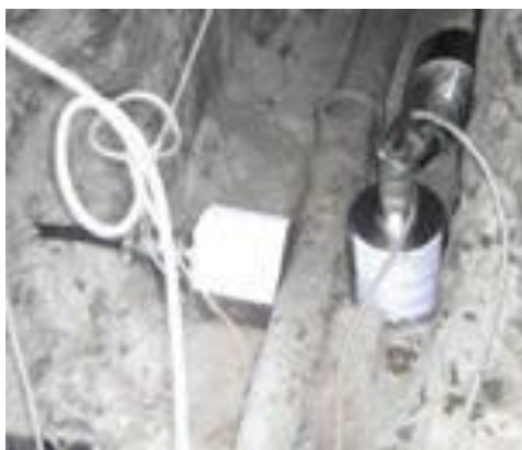
Fig. 5 – Vibration sensors № 1, № 2, № 3 for foundation oscillations registration towards X, Z and Y directions
