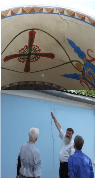
Fig. 2. Church's reaction to the explosion in the quarry. Top – cracks in the brick vault of the Church. Bottom – the priest pointing out vertical cracks on his house located within the Church's premises
