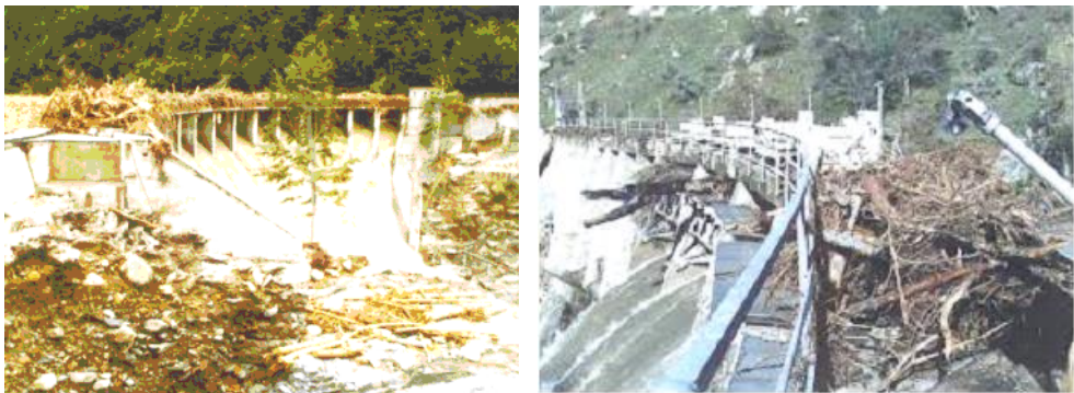
Fig. 2 – Overtopping of Palagnedra dam in Switzerland due to plugging of spillway by floating debris in 1978 (left) [27]; the similar plugging of the spillway of Kerckhoff dam in California, USA, in 1997 (right) [28]
